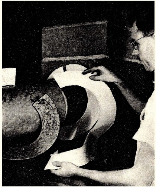
Left—When completed, this collar is not only efficient but has a neat appearance. Above—Several layers of asbestos are placed before the metal collar is fastened around the pipe.
